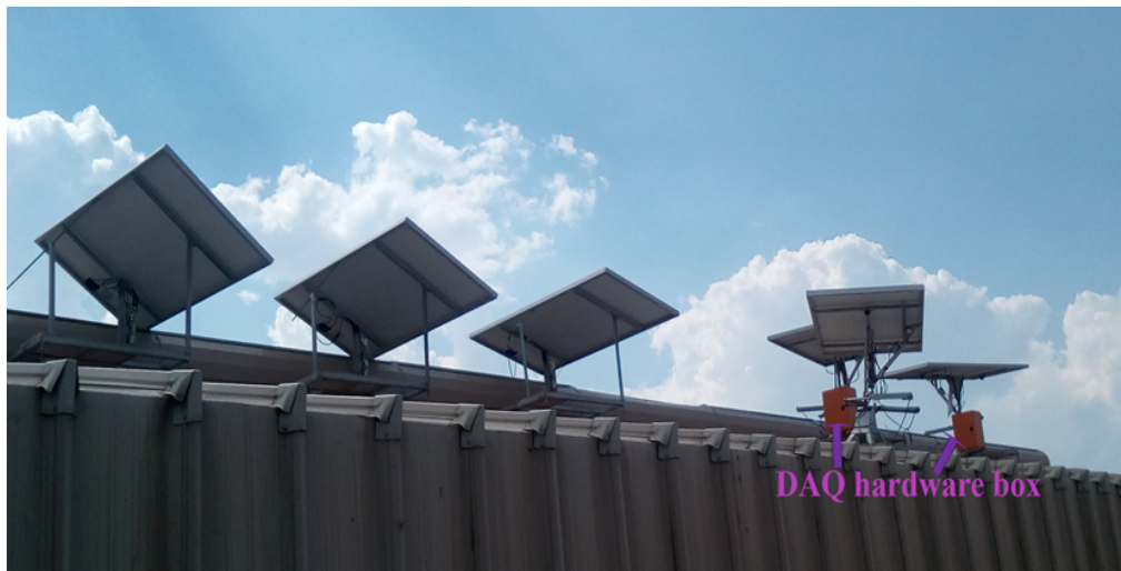
Figure 5. The DAQ system hardware box.
